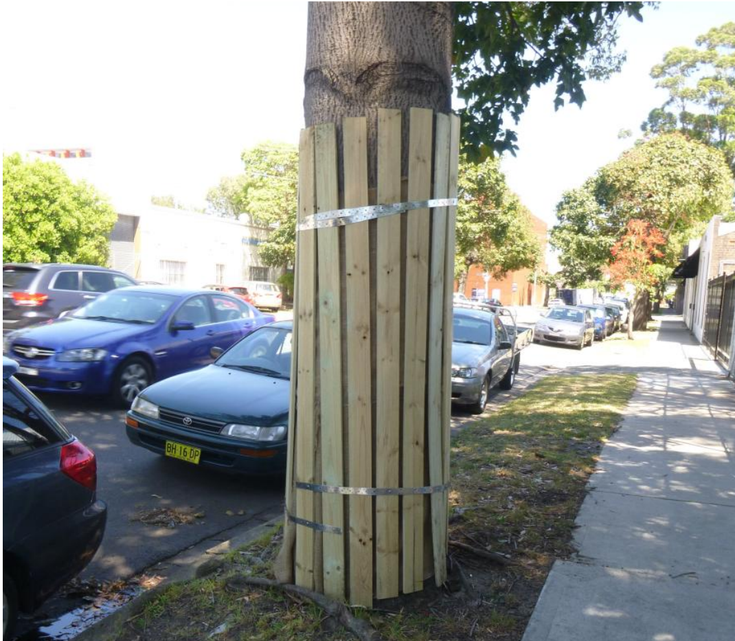
Figure 20 – Example of acceptable Trunk Protection batten installation
